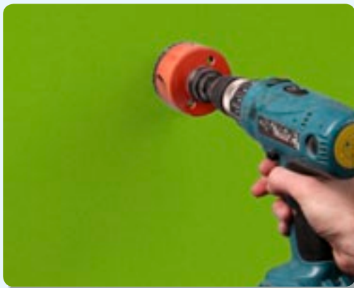
3. Drill a hole where the plug point is to be placed and install the wall socket.
